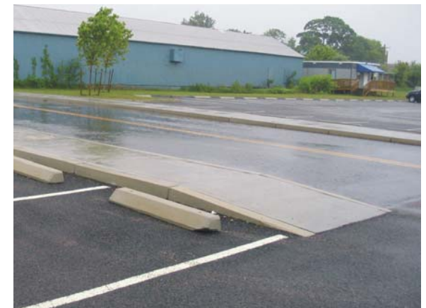
Rainwater infiltrates the porous asphalt yet accumulates on adjacent areas paved with conventional materials.
